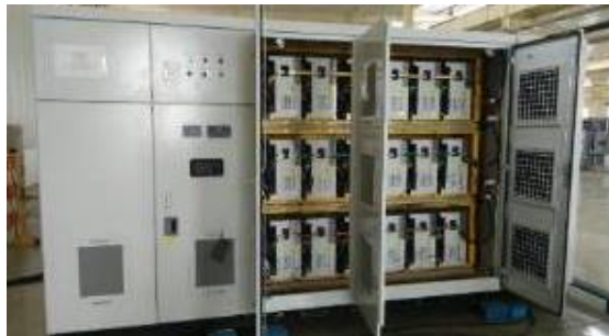
Fig. 12. 12-cell-cascaded 10 kV STATCOM
